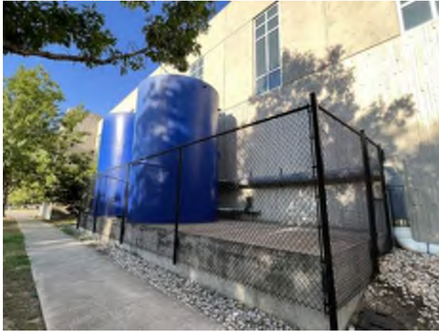
7. Rainwater collection tanks
