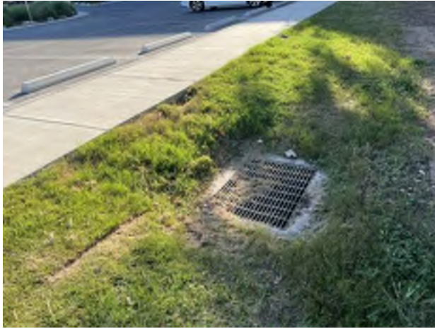
1. Catch basin at the landscaping.
