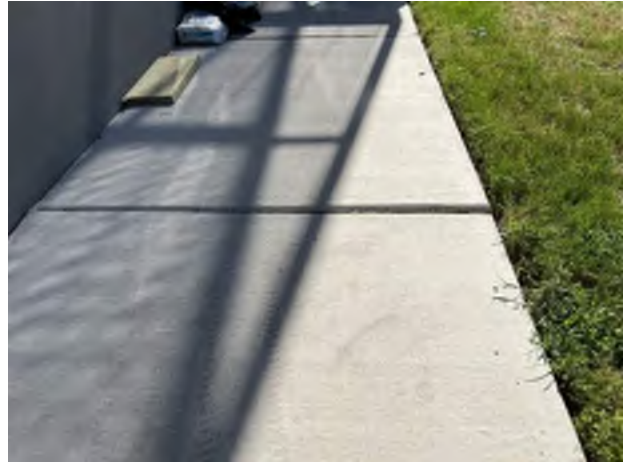
8. Settled concrete at the south walkway.
