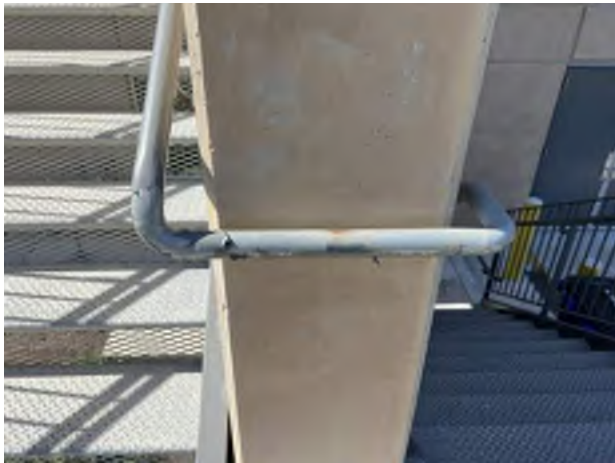
27. Chipped paint at north stairs.
