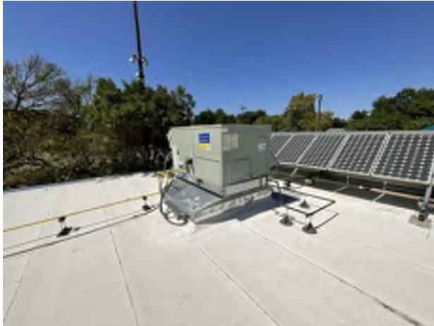
19. RTUs and Photovoltaic Panels
