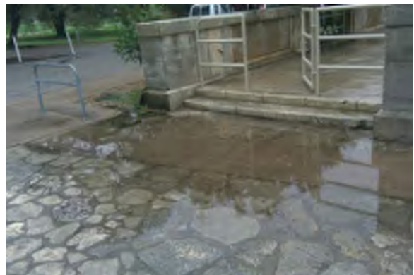
Figure 16. Poor drainage at northeast corner of the building
