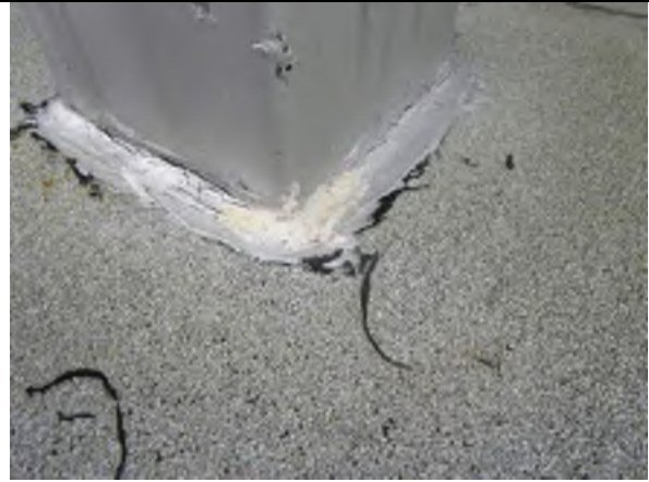
Sealant at the base of the pitch pan has failed and should be repaired with liquid applied membrane.
