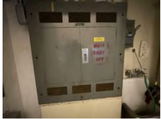
26. Main Disconnect Switch
