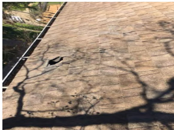
Damaged area needing decking replaced and roof restored to normal condition.
