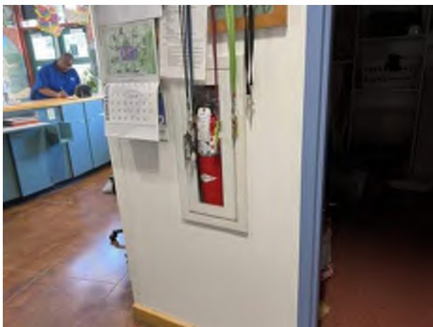
23. Manual fire extinguisher
