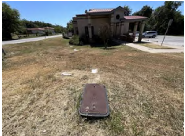
22. Water meter at the north side of the site.
