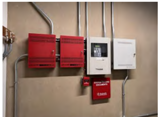
60. Fire alarm control panel.
