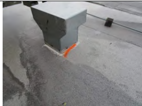
Abandoned T-top should be removed and roof brought back to original condition.
