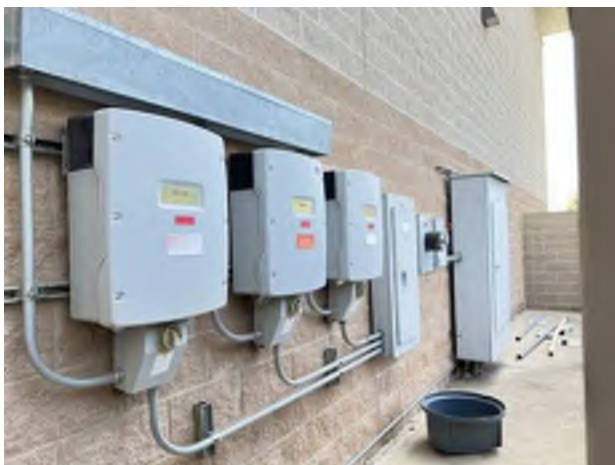
53. Main Building: Solar panel power inverters.
