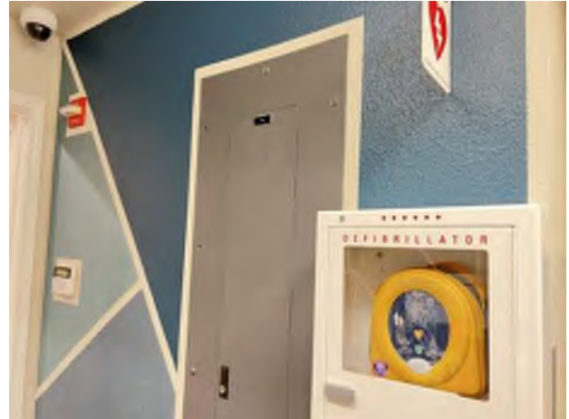
32. Electrical distribution panel.
