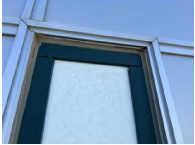
8. Failing Clerestory Window Sealant
