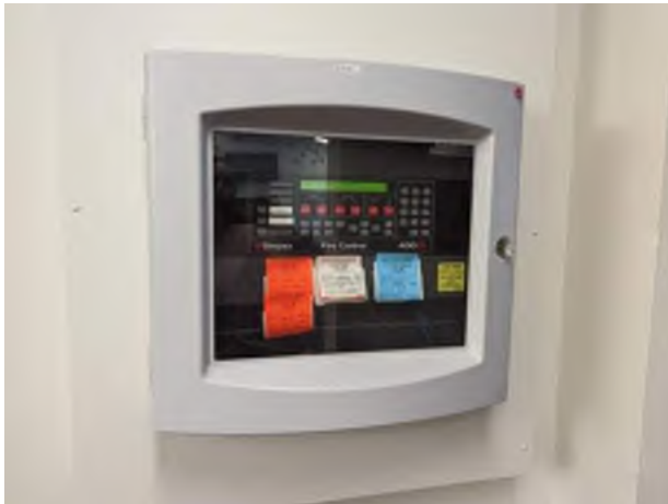
27. Fire Alarm Control Panel
