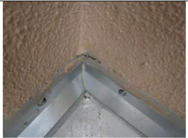
Caulking along existing counter flashing has failed and should be replaced with new sealant.
