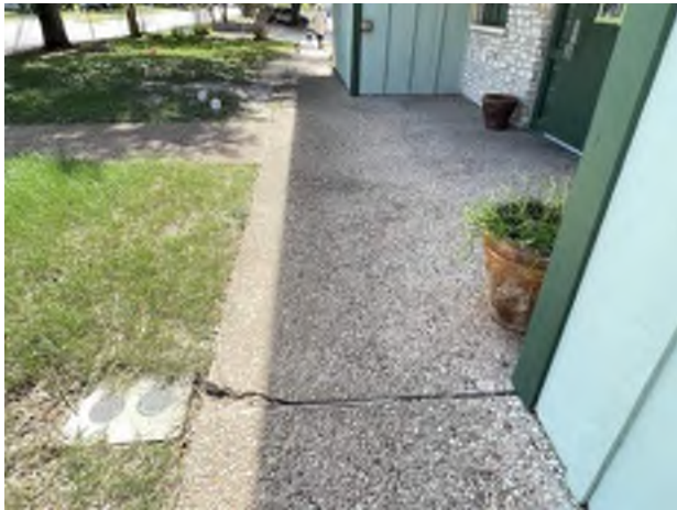
3. Cracked walkway - north side
