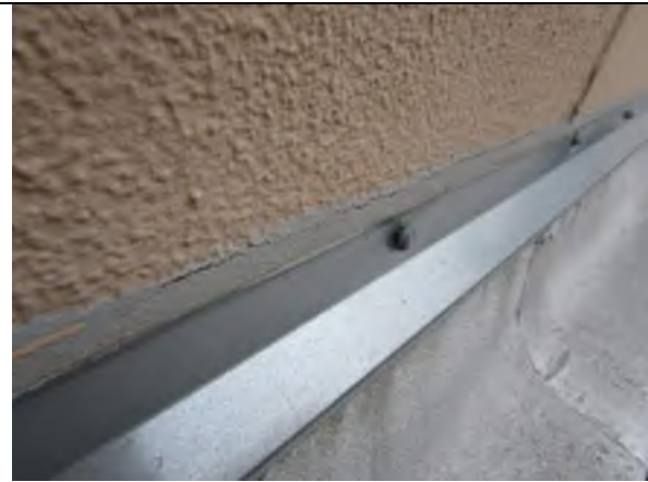
Caulking along existing counter flashing has failed and should be replaced with new sealant.
