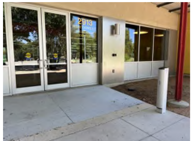
36. Automatic door opener at main entrance
