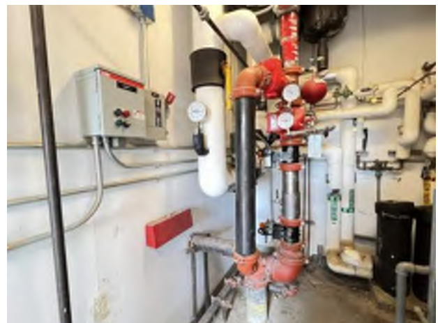
60. Main Building: Fire riser.
