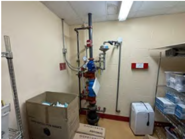
21. Fire Sprinkler Piping
