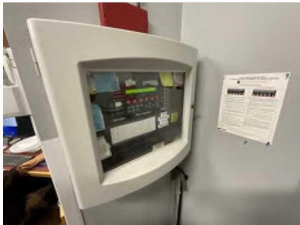
33. Main Fire Alarm
