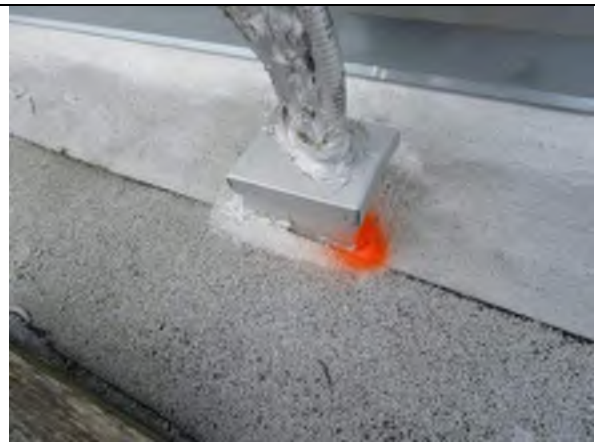
Pitch pan has failed and should be replaced.
