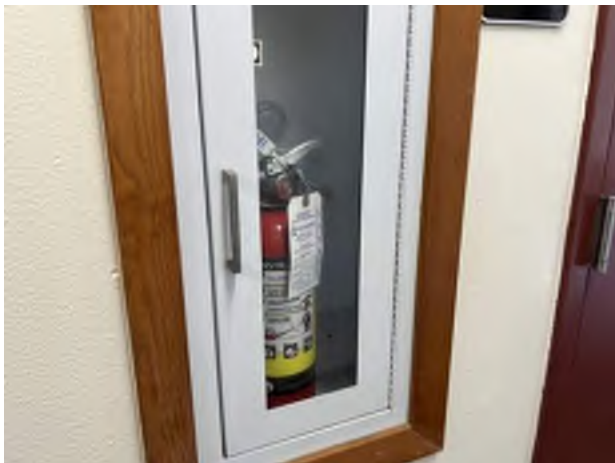
27. Recessed fire extinguisher cabinet.
