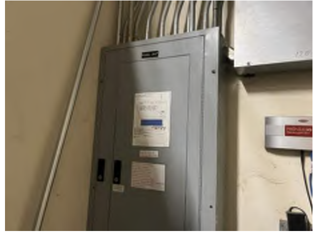
26. Electrical distribution panel.
