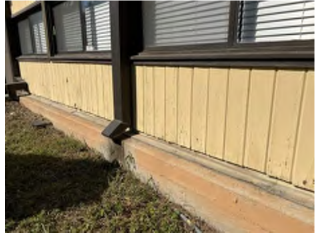
2. No splash block at east downspouts
