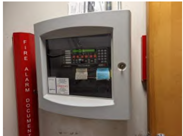
28. Fire Alarm Control Panel
