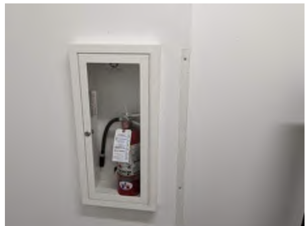
30. Fire Extinguisher in Recessed Cabinet
