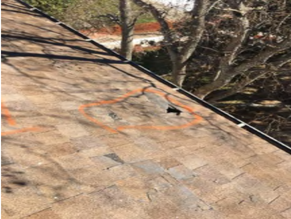
Damaged area marked.
