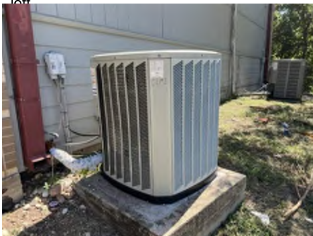
23. Condenser units at the west side of the building
