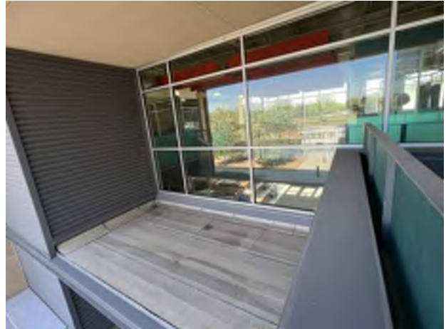
20. Windows and roofing at the west entry.
