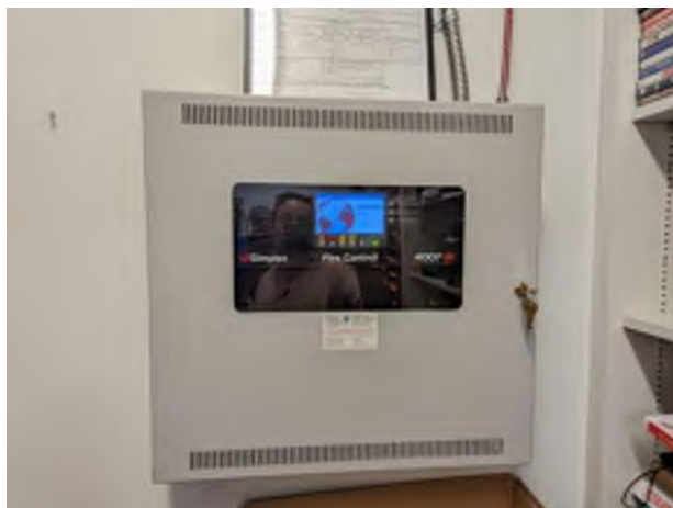
29. Fire Alarm Control Panel
