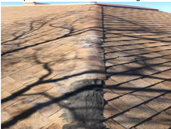
Ridge area needing repairs and ridge row replaced.
