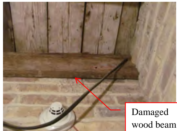
Figure 5. Beam damage under stair
