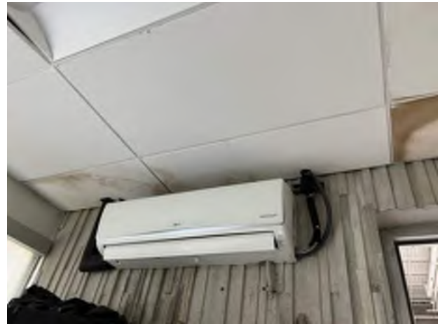
34. Split system air conditioner
