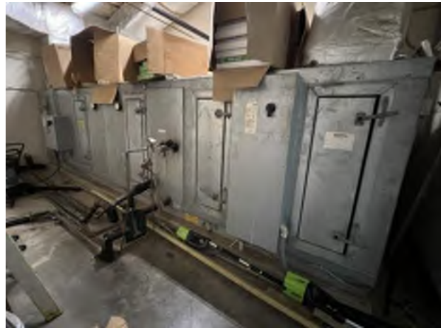
22. Energy recovery unit.
