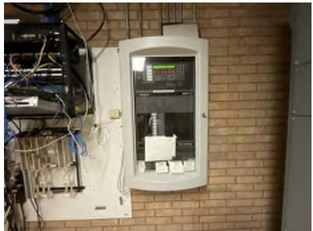
22. Fire Alarm Control Panel
