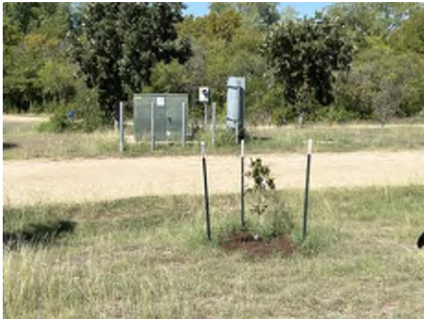
39. Transformer and Electrical Meter
