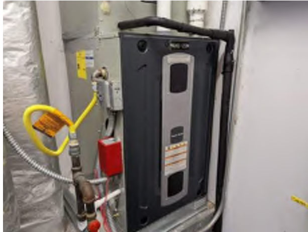
25. Air Hanlder Unit (Split System)
