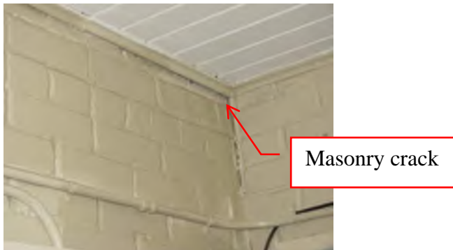
Figure 12. Masonry crack at ceiling in Teen Room
