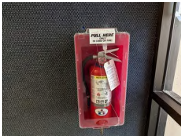
29. Typical Fire Extinguisher
