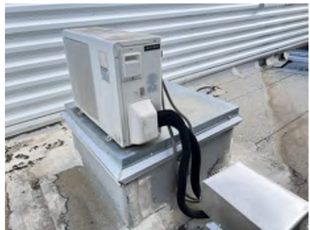
48. Main Building: Mini split system
