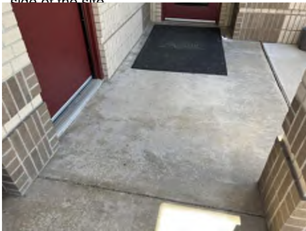
3. Isolated cracking at the concrete entryway.
