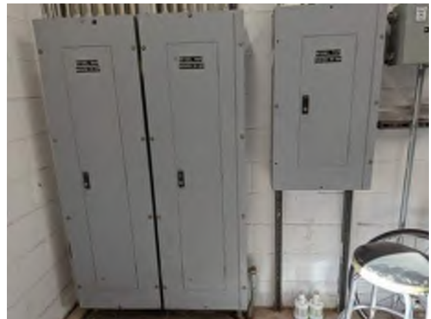
28. Main Electrical Panels
