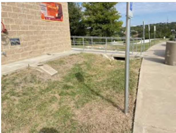
5. Multi-purpose Building: Drainage
