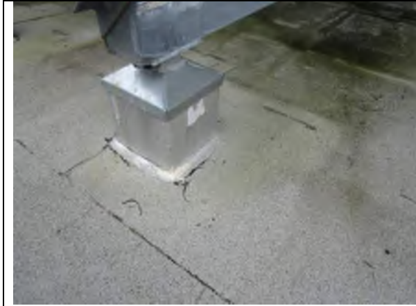
Sealant at the base of the pitch pan has failed and should be repaired with liquid applied membrane.
