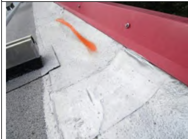
Blister in the existing base flashing. Blister should be cut out and roof repaired using modified bitumen.
