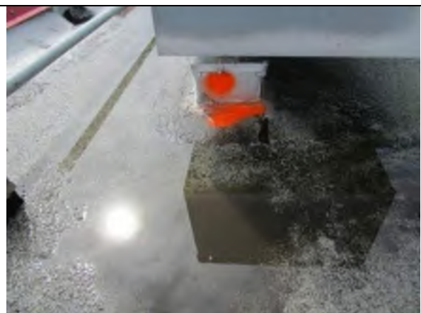
Sealant at base of existing pitch pan has failed and should be repaired using liquid applied membrane.
