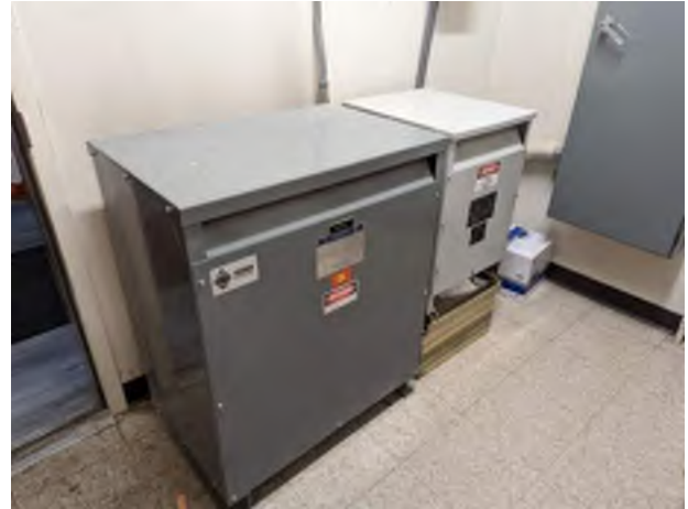
26. Interior Transformer 0 Main Building
