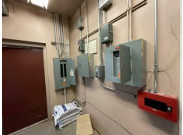
32. Circuit Breaker Panels
