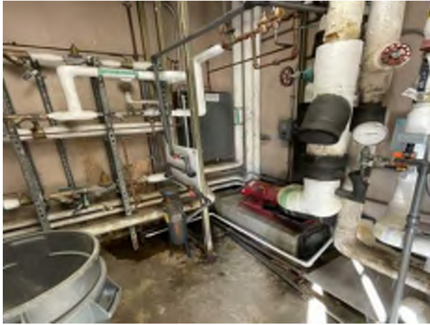
25. Chiller Pump Room
