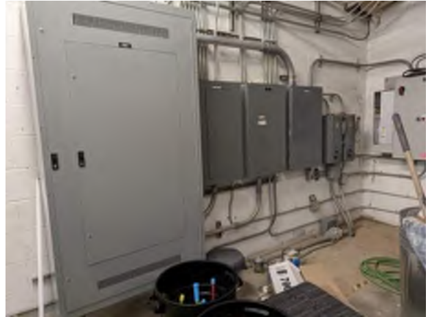
26. Interior Distribution Panels
