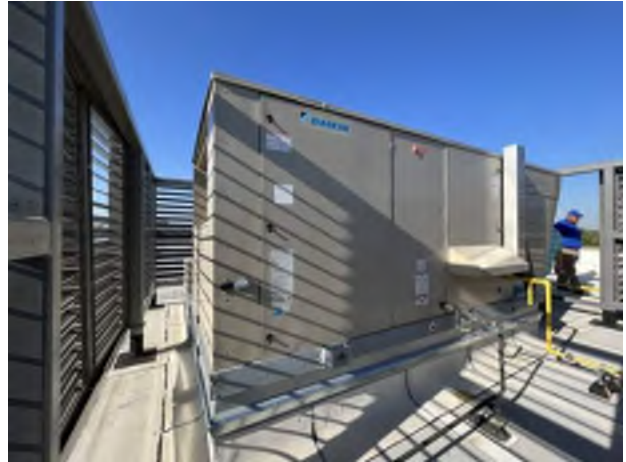
50. RTU-1 at the middle roof.
