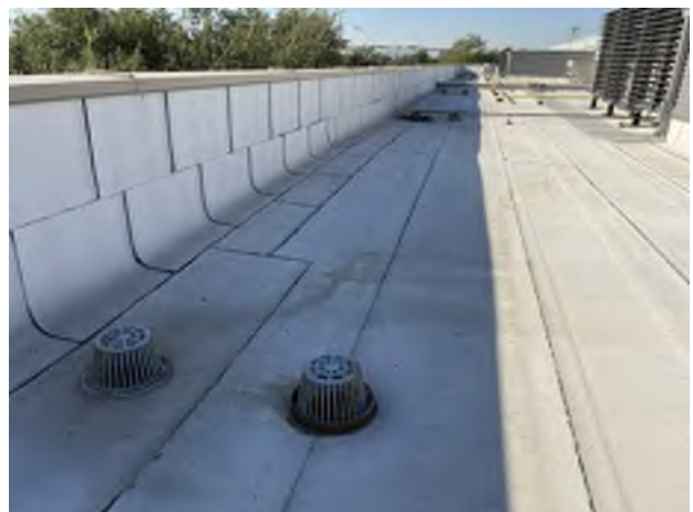
24. Roof and overflow drains.
