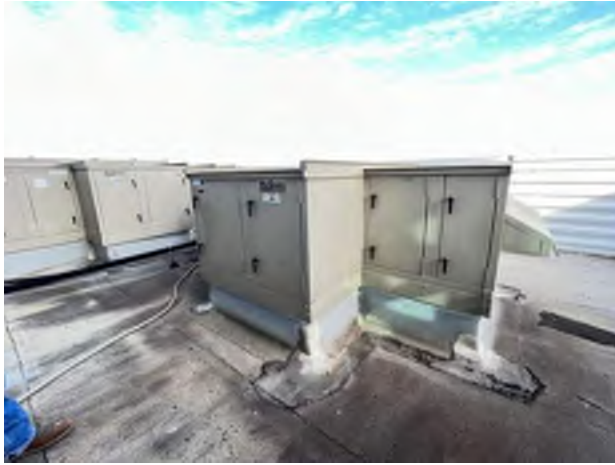
49. Main Building: Fan coil units
