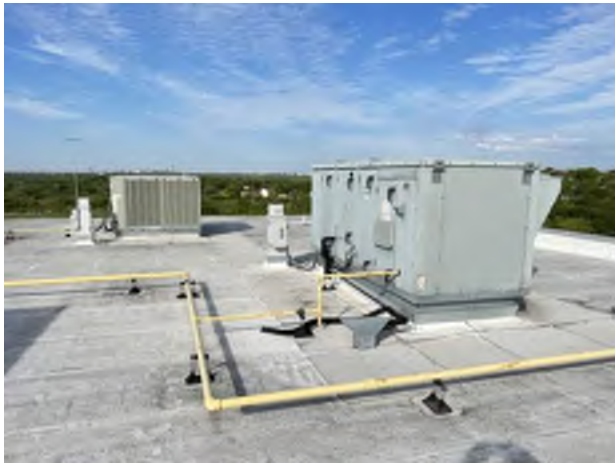
51. RTU at Main Building
