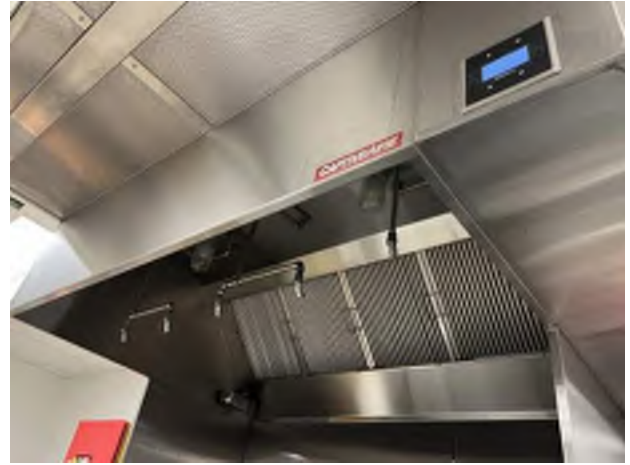
62. Kitchen hood with fire suppression.
