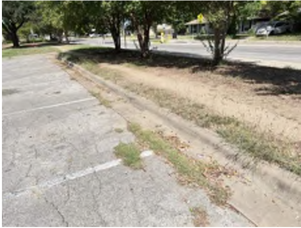
1. Vegetation and debris at the concrete gutter.
