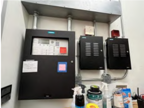
37. Fire alarm control panel
