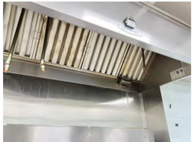
64. Ansul system at the kitchen hood.
