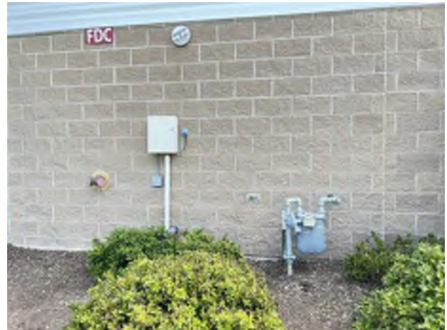
46. Main Building: Gas meter
