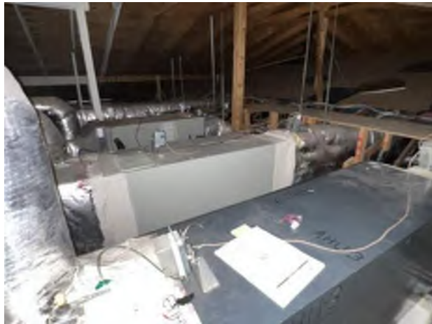
27. Mechanical loft at the attic space.
