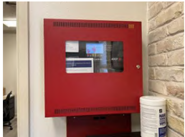
28. Fire alarm panel
