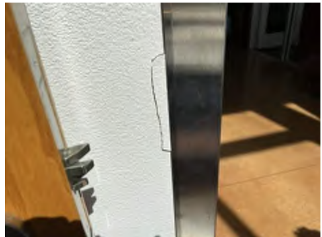
28. Damage at Entry/Exit Door
