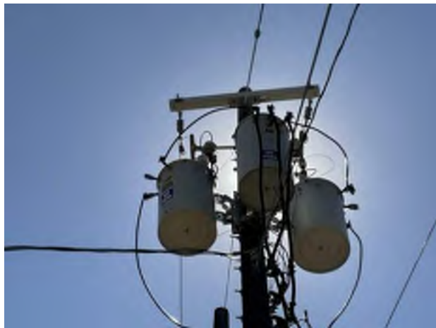
21. Transformers Feeder Pole
