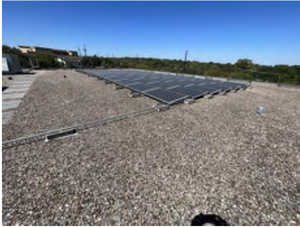
31. Solar panels at the upper roof
