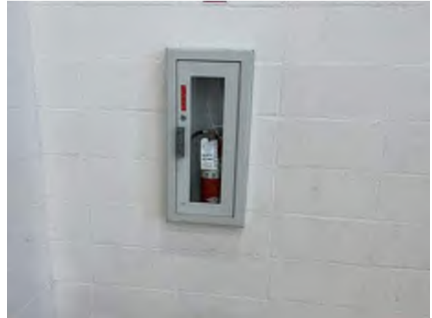
44. Recessed Fire Extinguisher Cabinet
