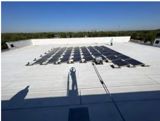
57. Solar panels at the upper roof.
