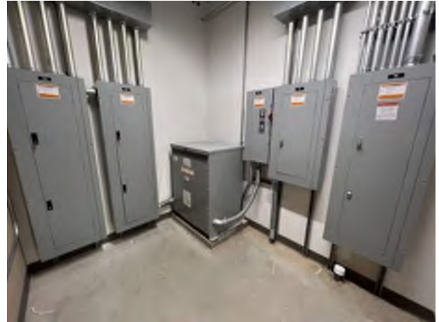
56. South electrical room.
