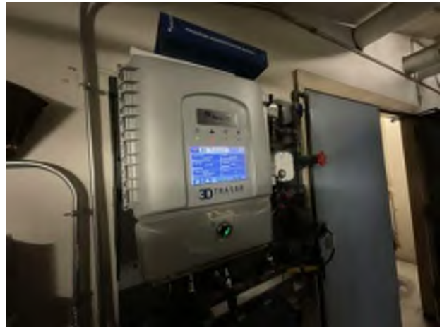
28. Water Management Monitoring System
