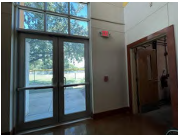
29. Illuminated exit sign and fire alarm pull.
