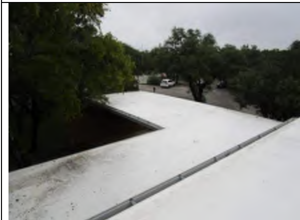
Sealant around hot stack has failed and needs to be replaced.
