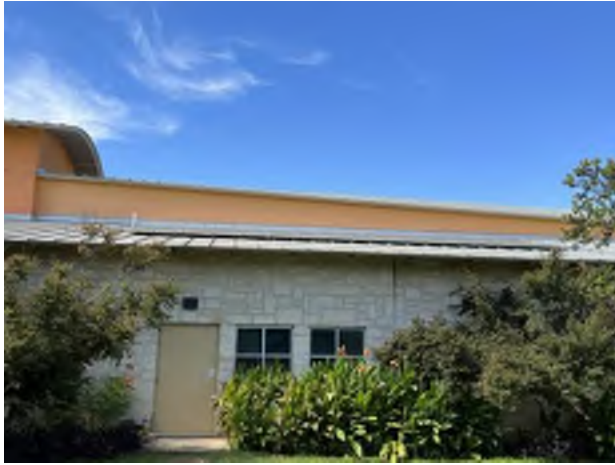
25. Solar panels at the roof.
