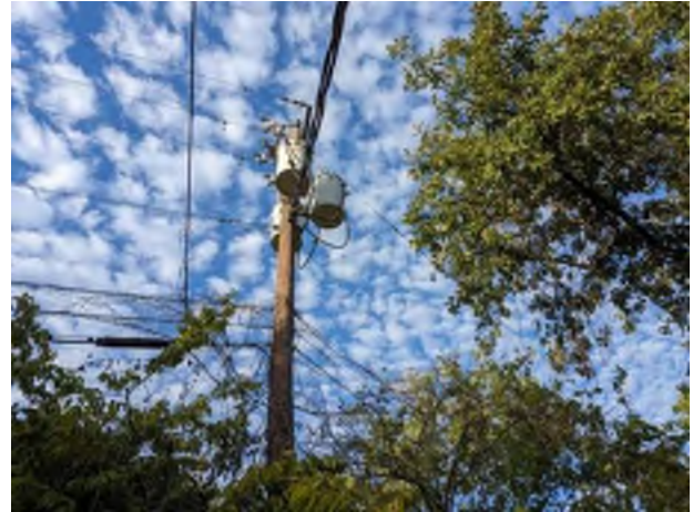
26. Pole Mounted Transformer
