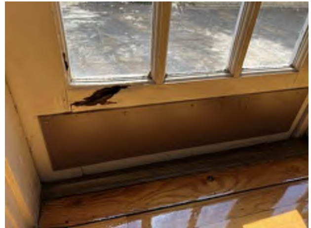
10. Damaged exterior door
