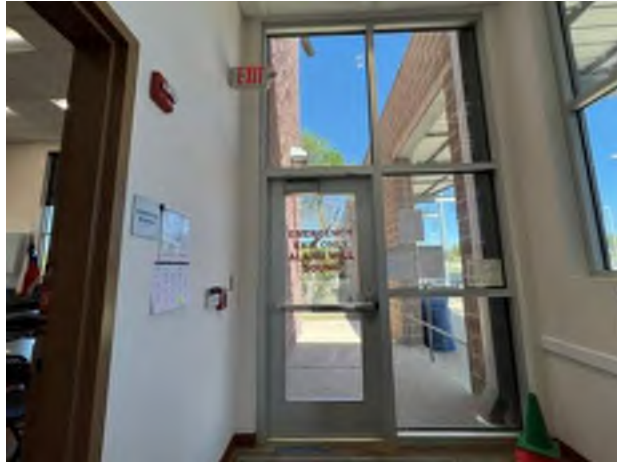
43. Illuminated Exit Sign and Fire Alarm Strobe
