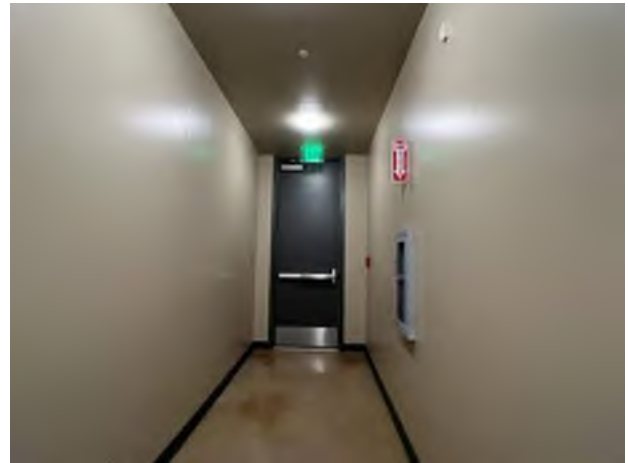
34. Exit sign and fire extinguisher
