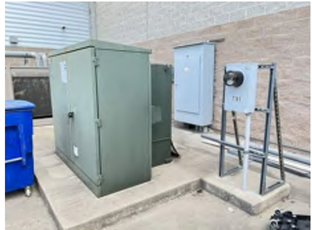
52. Pad mounted Transformer
