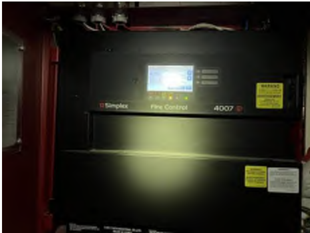
27. Fire alarm control panel
