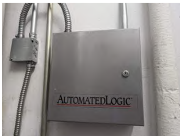
23. Building Automatic Panel
