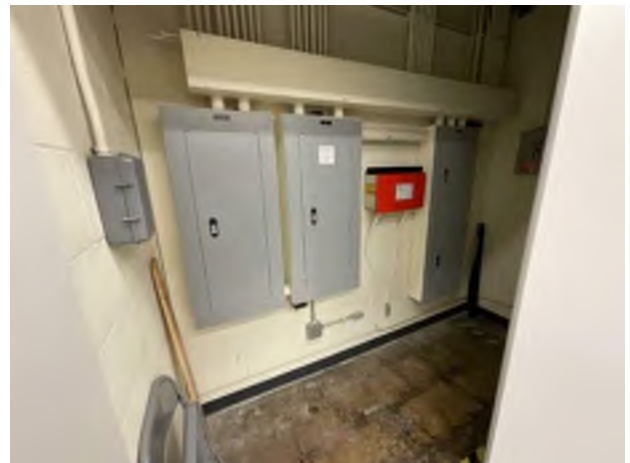
22. Main Electrical Panel
