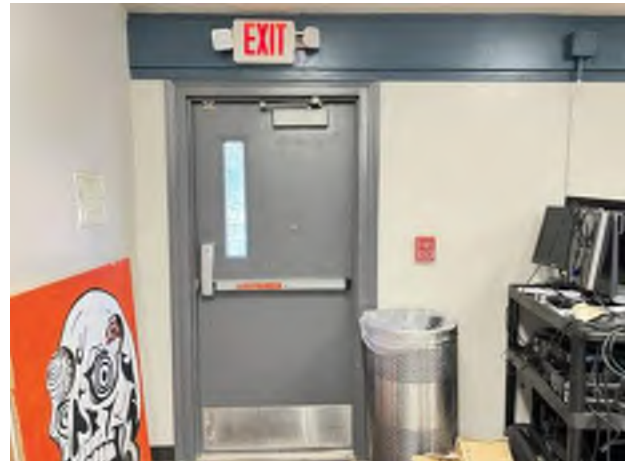
34. Exit Sign and Fire Alarm Pull
