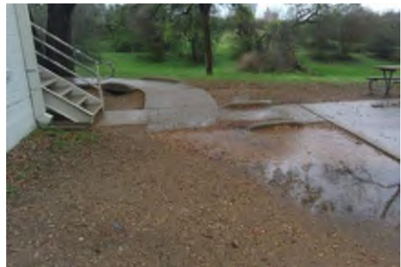
Figure 15. Poor drainage at west end of building
