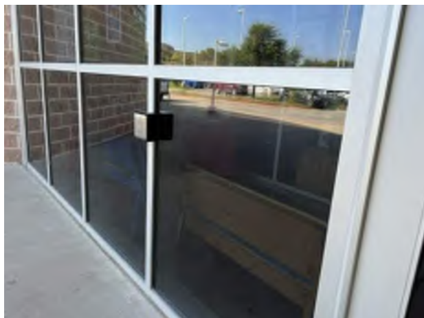
47. Automatic Entry Door Operator
