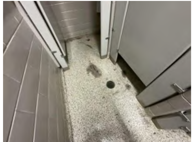
22. Bathroom Not ADA
