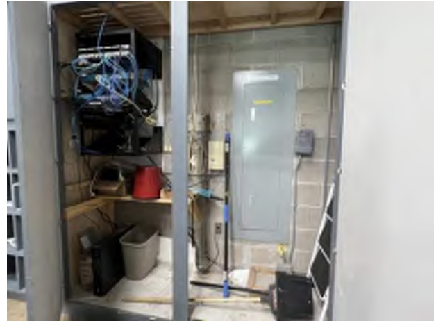
26. Main distribution panel.
