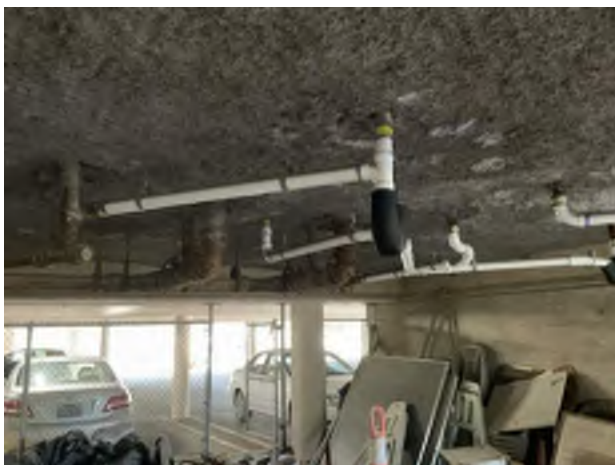
23. Waste Water Pipe
