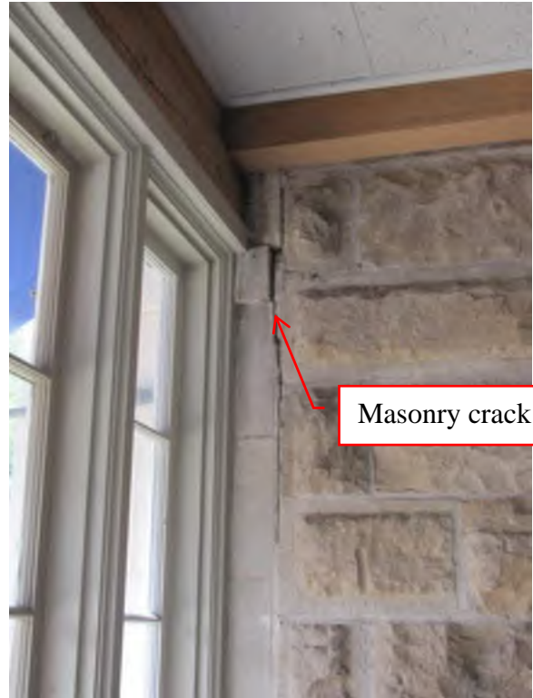
Figure 4. Masonry crack at Sun Porch southwest corner
