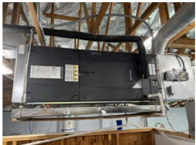
24. Air handler unit at the mechanical loft.
