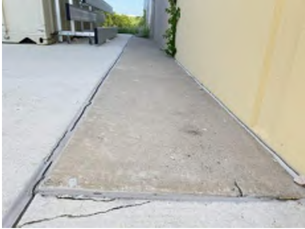
13. Settlement at Main Building
