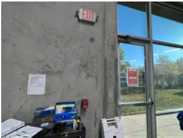
39. Illuminated exit sign and fire alarm pull
