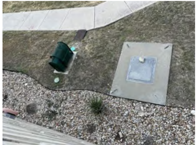
28. Water meter and backflow preventer
