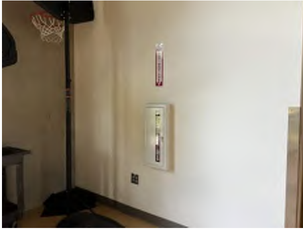
61. Recessed fire extinguisher cabinet.
