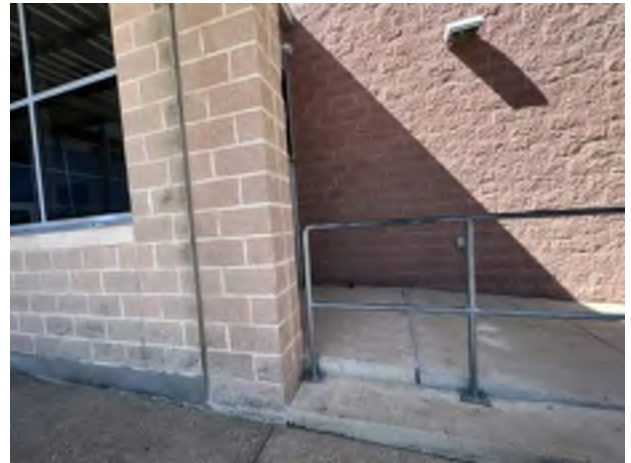
4. Patched Brick course and some efflorescence
