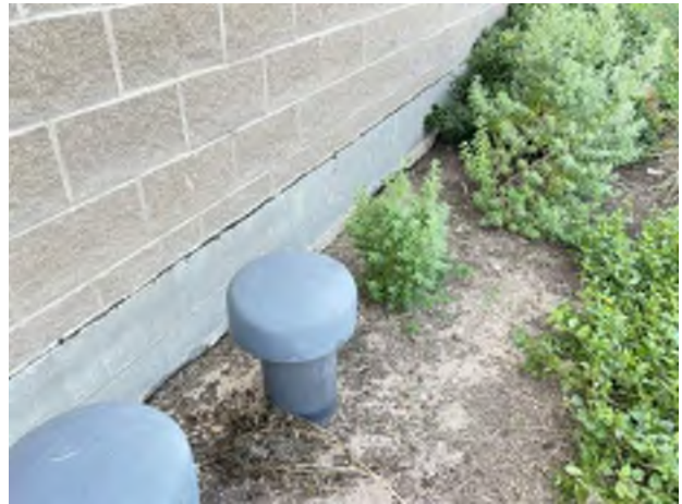
4. Main Building: Settlement north side
