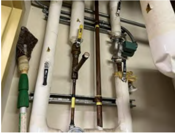
19. Domestic water supply.
