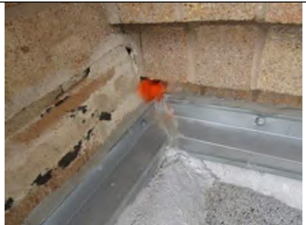
Mortar joint has opened. Sealant should be installed to prevent water intrusion.
