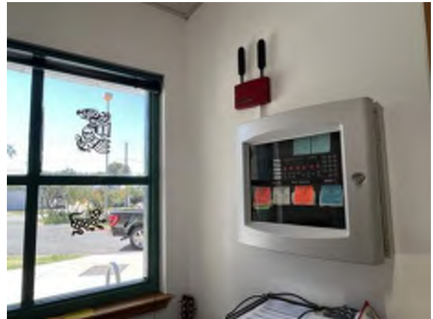
22. Fire alarm panel
