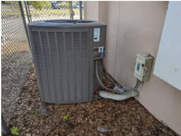
21. Typical Condenser (Main Building)
