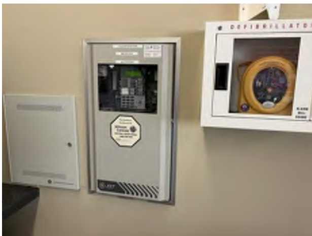
35. Fire alarm panel
