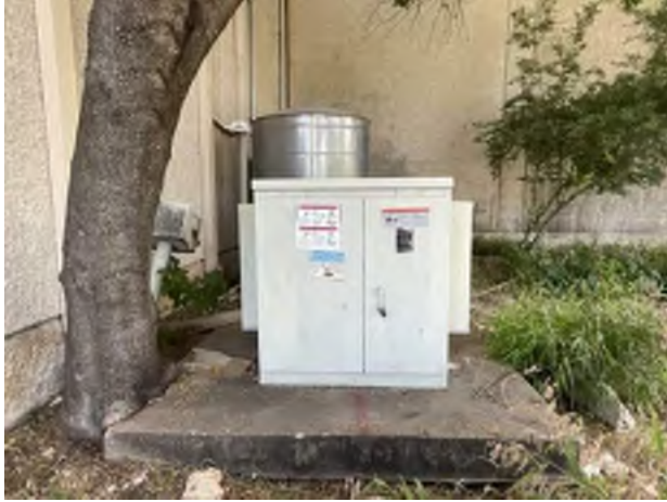
25. Utility Owned Transformer
