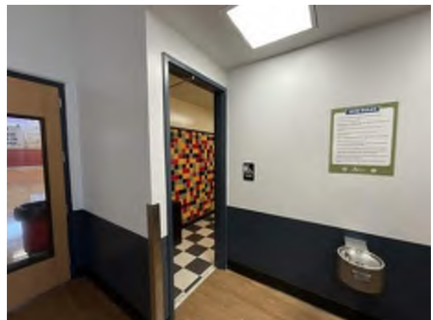
30. Drinking Fountain limits accessibility to both restrooms
