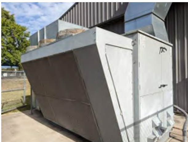
23. RTU at Gym
