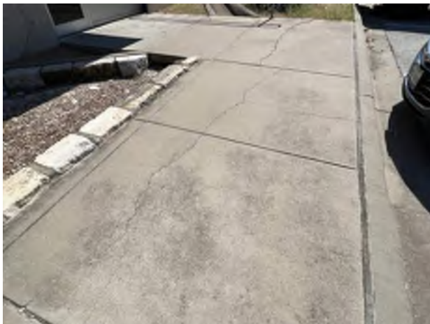
5. Cracked concrete walkway
