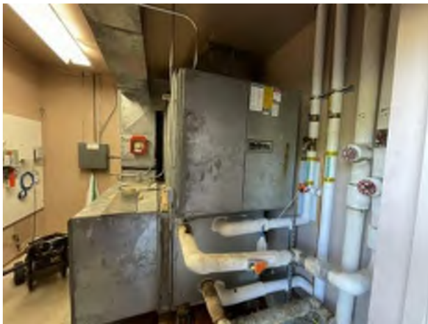
27. Central System Air Handler
