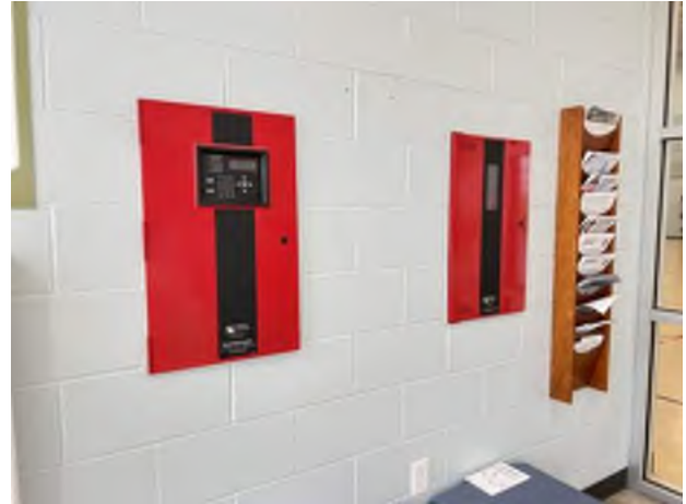
62. Multi-purpose Building: FACP
