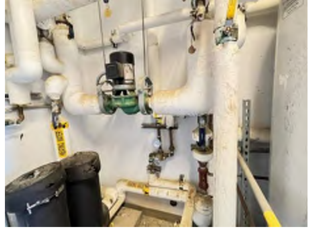
44. Main Building: Domestic water supply.
