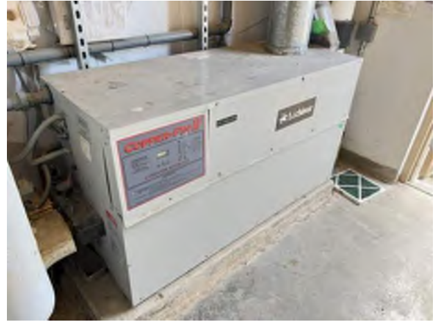
50. Main Building: Boiler.
