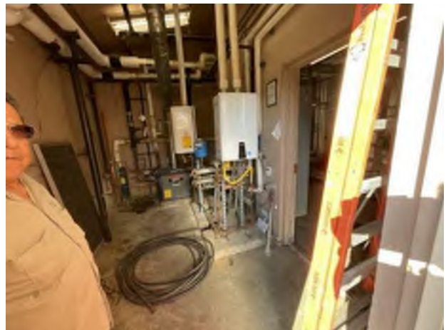
24. Boiler and Water Heaters
