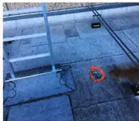
Old Patch needing properly repaired.
