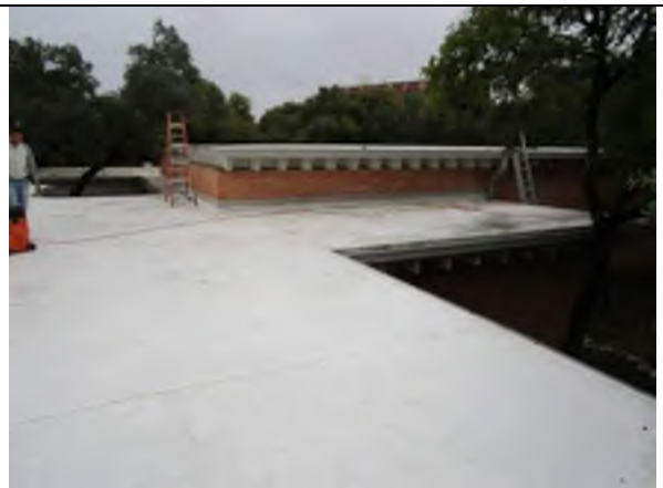
Sealant around pipe boot has failed and needs to be replaced.
