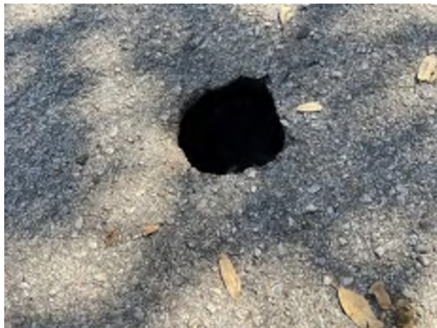
3. Sinkhole at lower parking lot
