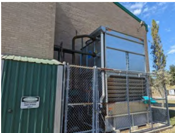
23. BAC Cooling Tower
