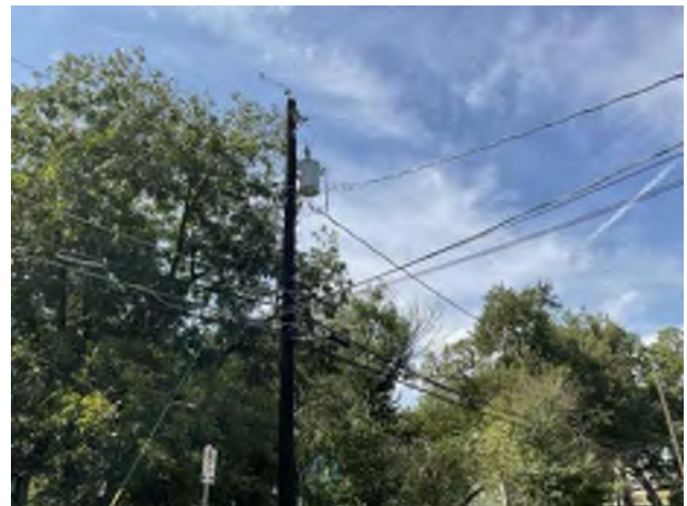
28. Pole Mounted Transformer
