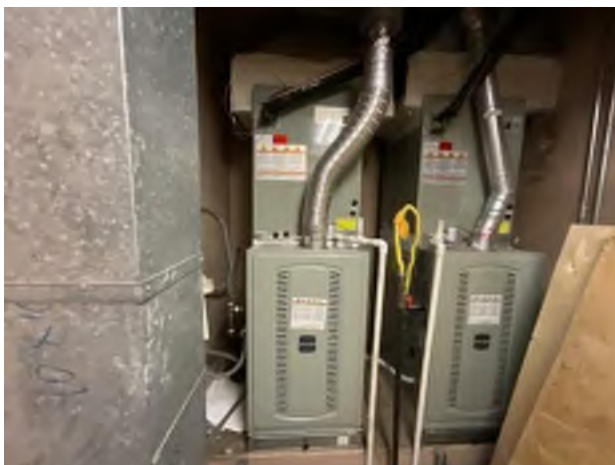
29. Split System AHUs
