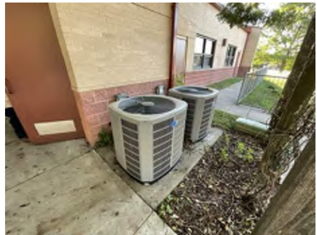
28. Split System Condensing Units
