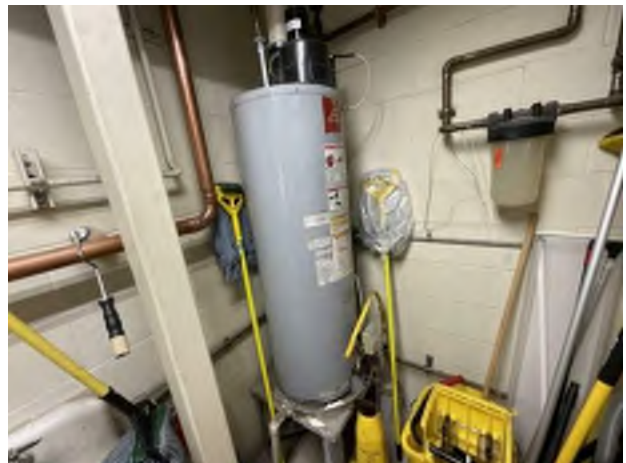
18. Gas Water Heater
