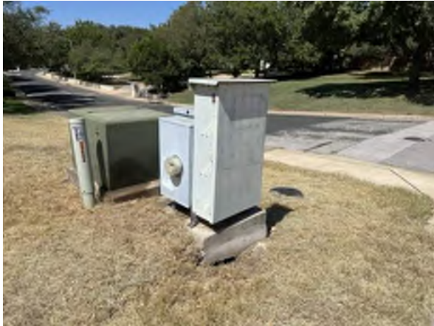
25. Transformer and electrical meter.
