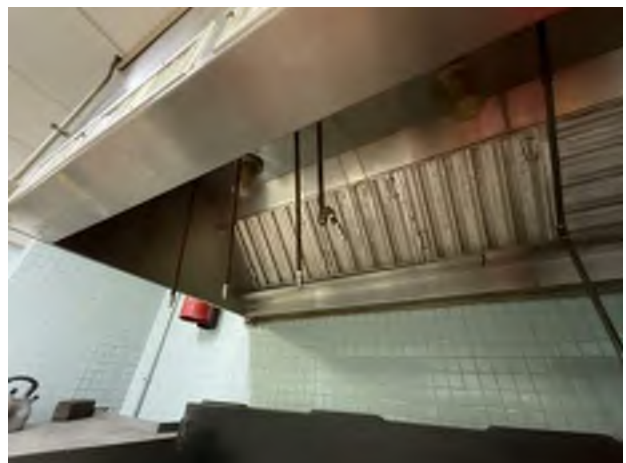
36. Hood and Ansul system
