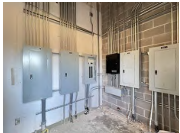
54. Electrical distribution panels.
