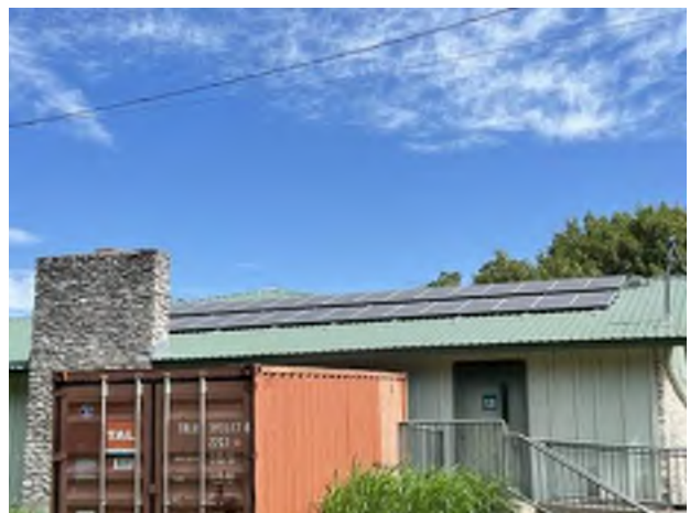
30. Solar panels at the roof.
