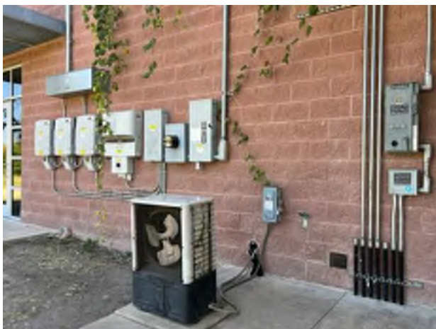
41. Solar Power Inverters
