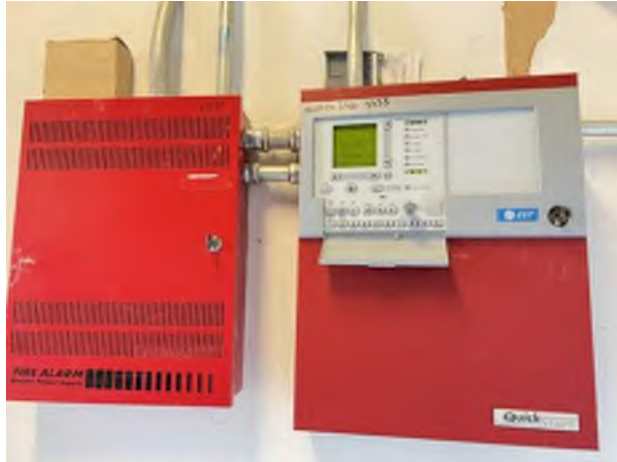
61. Main Building: Fire alarm control panel.
