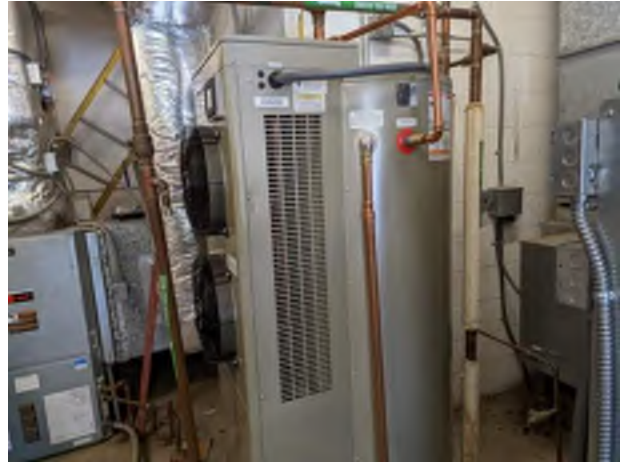
20. Hot Water Heater
