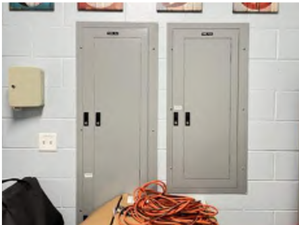
57. Multi-purpose Building: Electrical panels.
