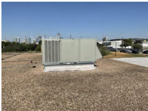
17. Roof top unit (typical)
