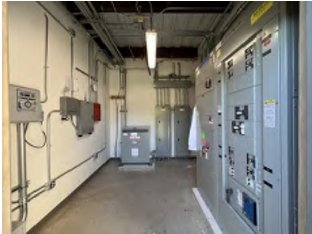
55. North electrical room.
