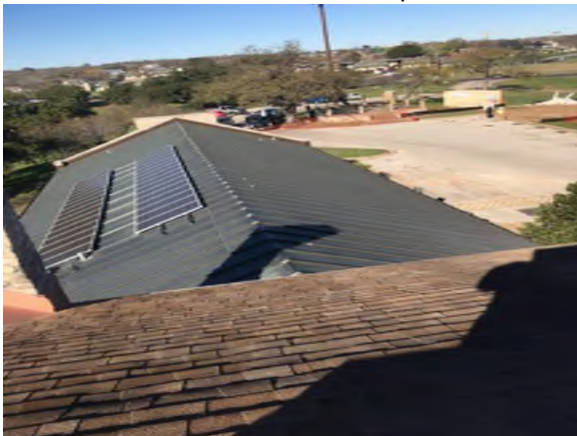
Overview of Metal roof area. Also showing the (3) penetrations needing replaced, one close to solar panels and 2 at the far end on right.
