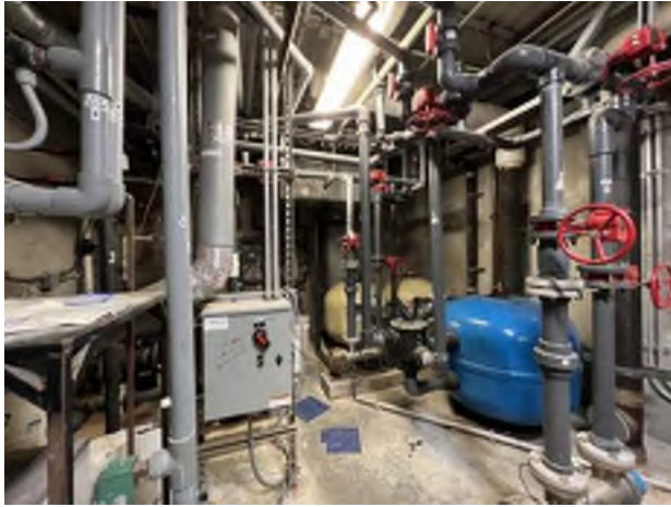
31. Pool equipment room
