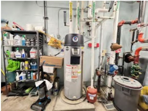
45. Multi-purpose Building: Water heater.
