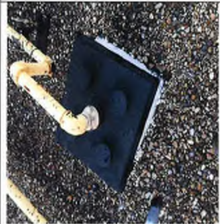
Gas line needing to be sealed.
