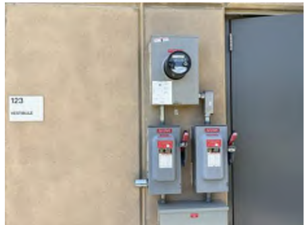
58. PV electrical meter.
