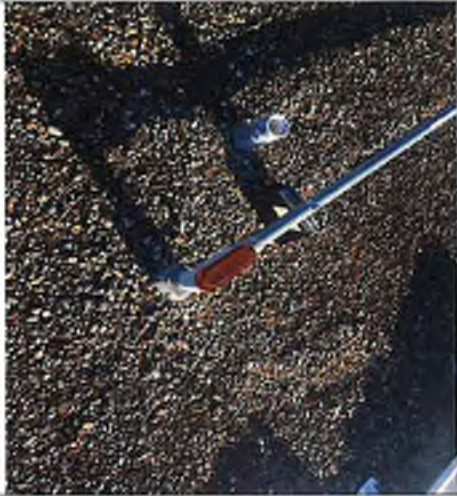
New sealant needed.
