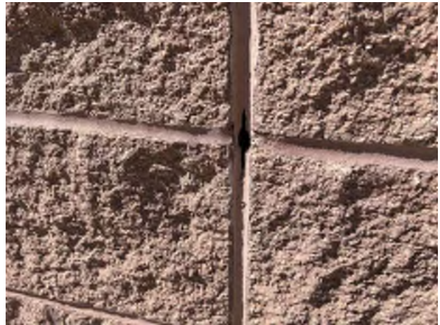
10. Failing Building Expansion Joint
