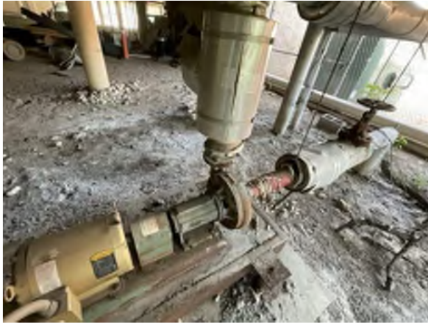
25. Cooling Tower Pump
