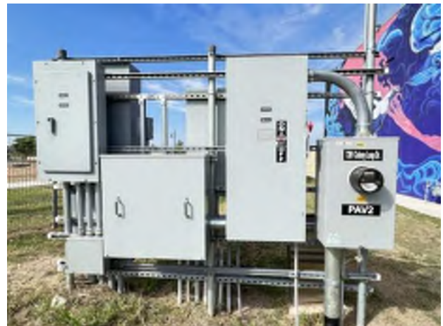
58. Multi-purpose Electrical panel
