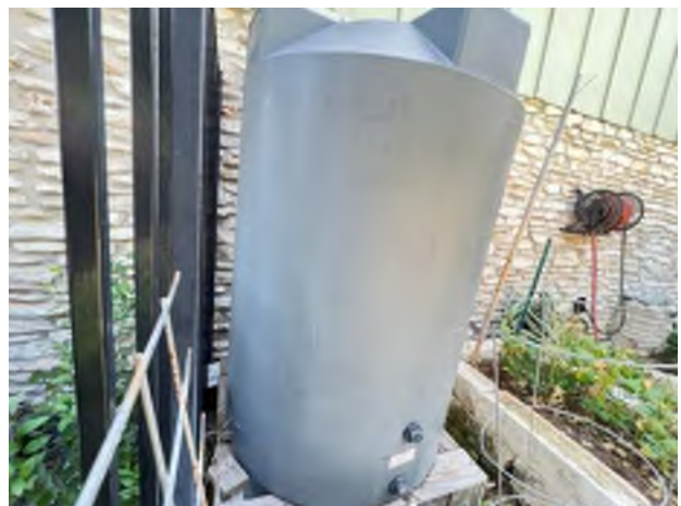
6. Rainwater collector for garden irrigation.
