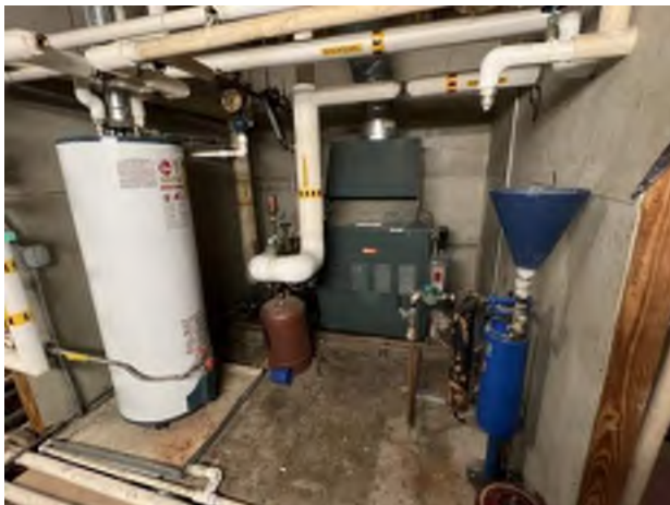
23. Water heater and boiler
