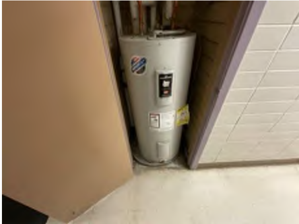
13. Subject: Water Heater
