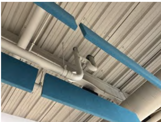
41. Leaking pipe at the ground floor ceiling.
