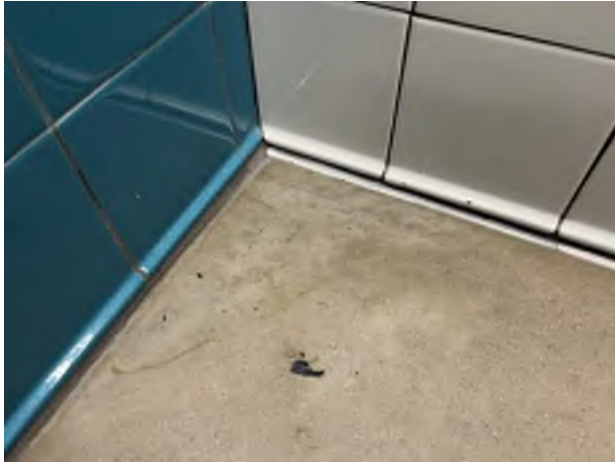
49. Recaulked joint at the shower room floor.
