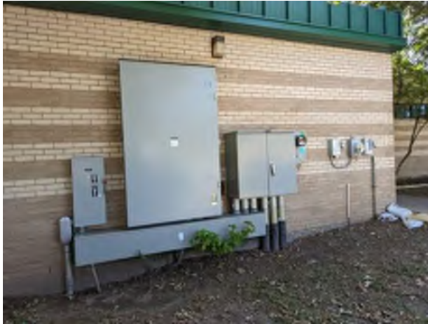
25. Electrical Switch and Meter
