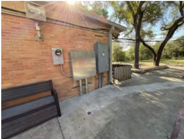
15. Subject: Main Electrical Panel
