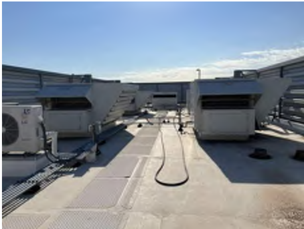
33. Rooftop mechanical yard
