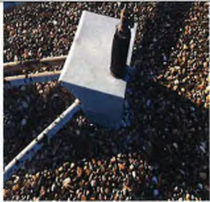
Close up of penetration in top of pitch pan.
