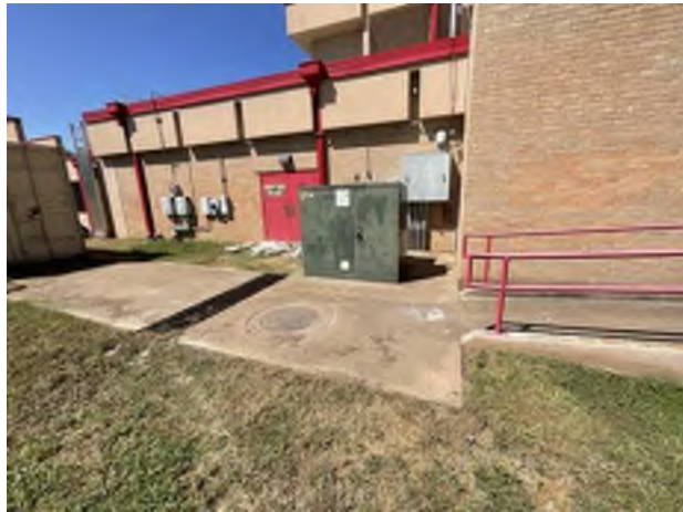
15. Transformer Pad and Worn Metal Door Paint
