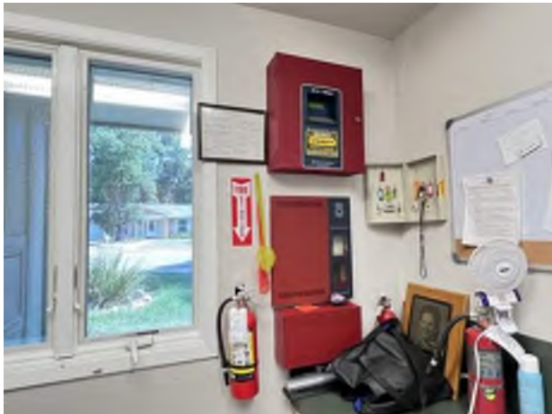
33. FACP and Fire Extinguisher
