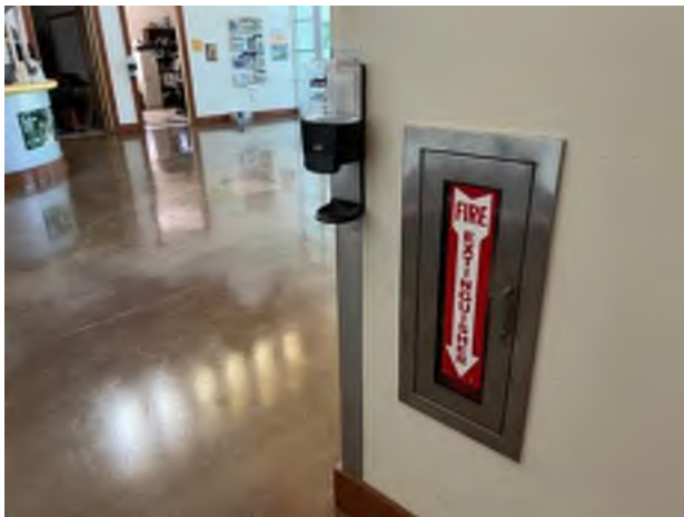
27. Recessed fire extinguisher.
