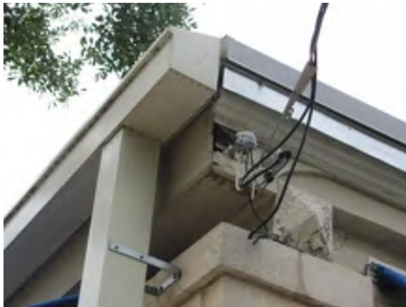
Figure 13. Eave damage at the southeast building corner
