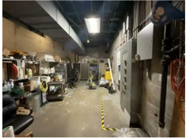
20. Gymnasium Electrical Room
