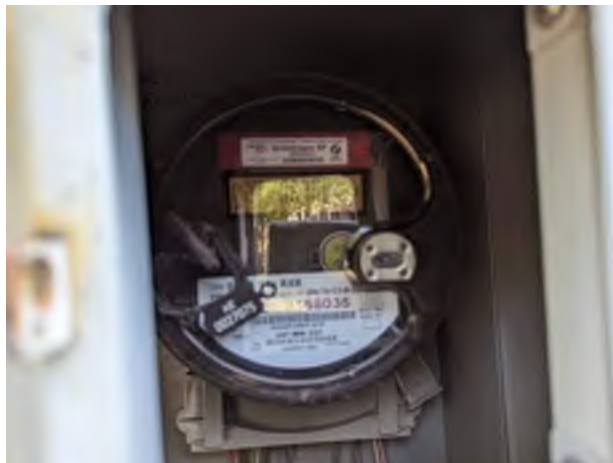
27. Electrical Meter on South Wall
