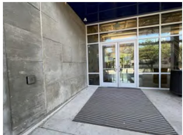
42. Automatic door opener at main entrance door
