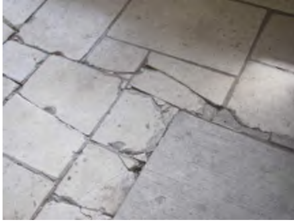
Figure 6. Sun Porch Floor damage
