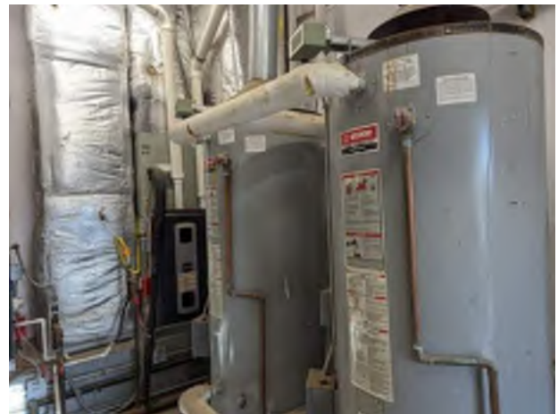
22. Hot Water Heaters
