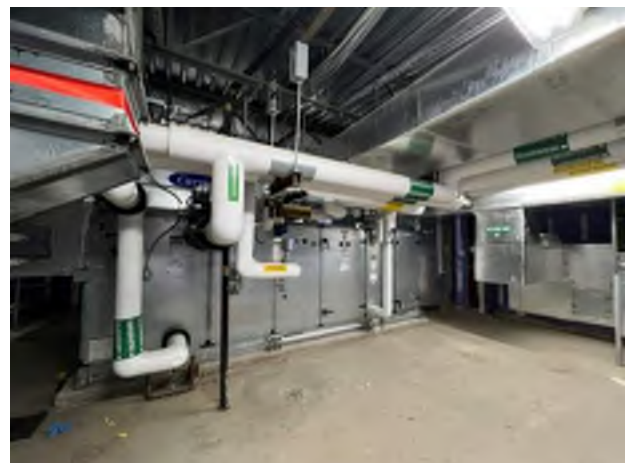
36. Air Handler Unit
