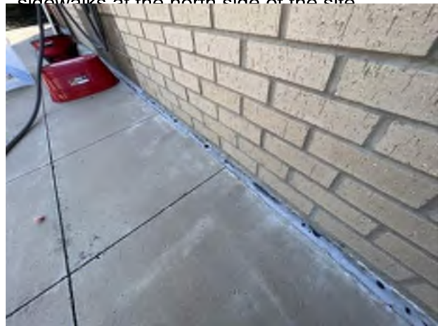
4. Failing expansion joint along the east building perimeter
