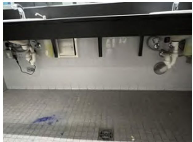
48. Insulated Pipes at Lavatories
