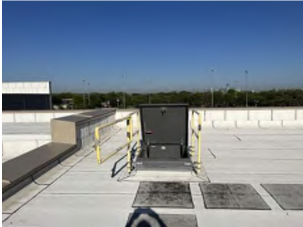
25. Roof hatch at the middle roof.
