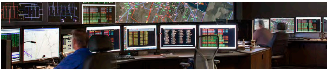
Austin Energy System Control Center
