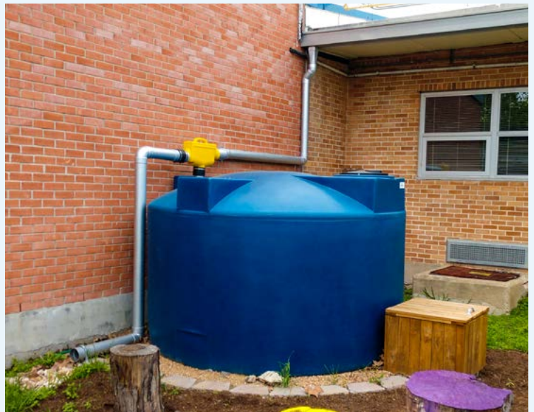
Figure 13b. Cistern being monitored at Reilly Elementary
