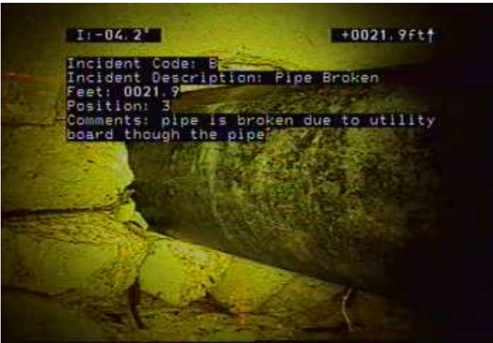
B - Pipe Broken @ 21.9 ft. pipe is broken due to utility board though the pipe
