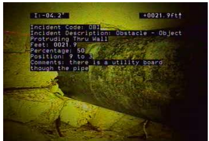
OBI - Obstacle - Object Protruding Thru Wall @ 21.9 ft. there is a utility board though the pipe
