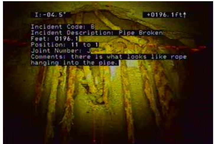
B - Pipe Broken @ 196.1 ft. there is what looks like rope hanging into the pipe.
