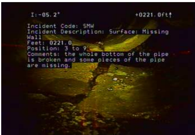
SMW - Surface: Missing Wall @ 221.0 ft. the whole bottom of the pipe is broken and some pieces of the pipe are missing.
