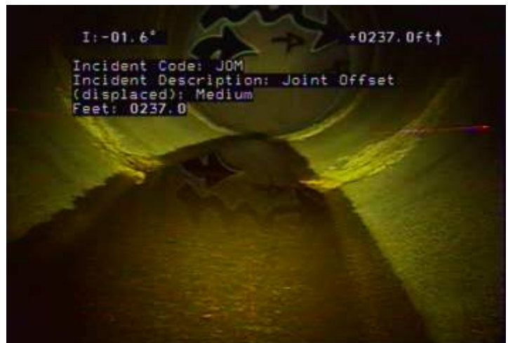
JOM - Joint Offset (displaced): Medium @ 237.0 ft.
