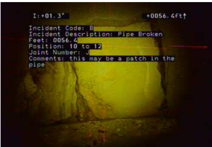
B - Pipe Broken @ 56.4 ft. this may be a patch in the pipe
