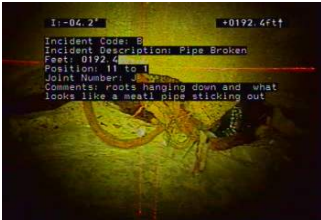
B - Pipe Broken @ 192.4 ft. roots hanging down and what looks like a meat pipe sticking out
