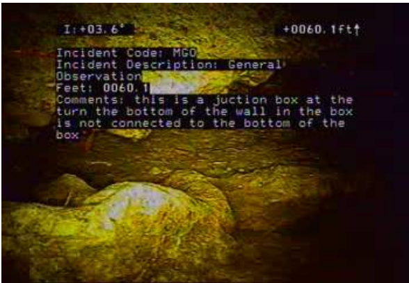
MGO - General Observation @ 60.1 ft. this is a junction box at the turn the bottom of the wall in the box is not connected to the bottom of the box
