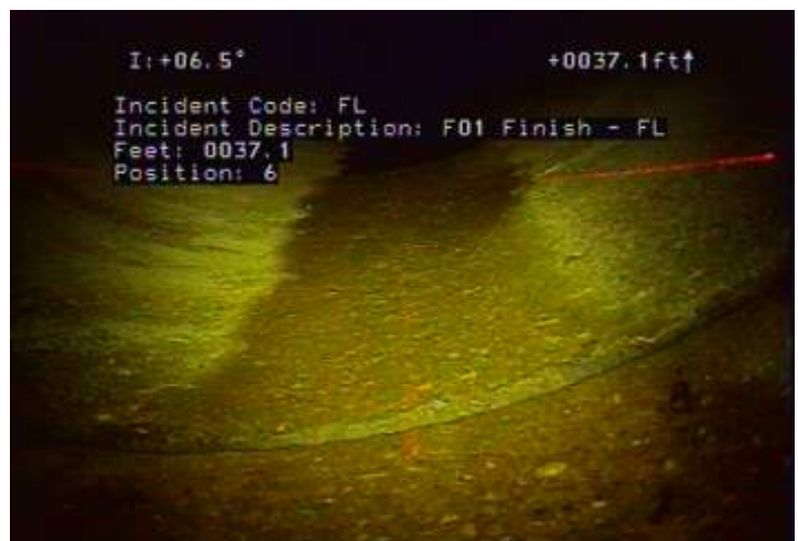
FL - Fracture Longitudinal @ 37.1 ft.
