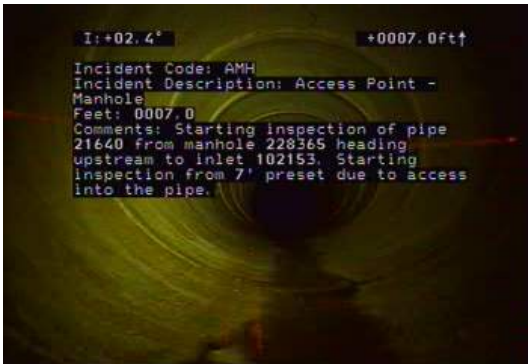
AMH - Access Point - Manhole @ 7.0 ft. Starting inspection of pipe 21640 from manhole 228365 heading upstream to inlet 102153. Starting inspection from 7' preset due to access into the pipe.
