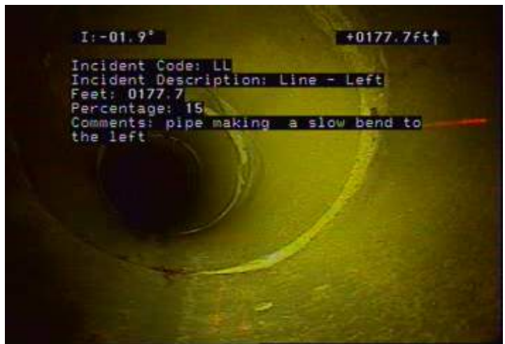
LL - Line - Left @ 177.7 ft. pipe making a slow bend to the left
