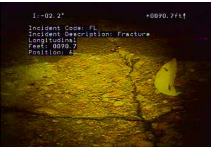
FL - Fracture Longitudinal @ 90.7 ft.
