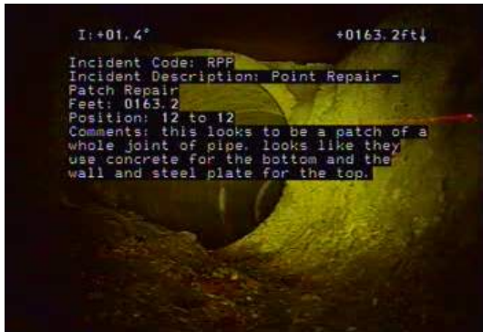
RPP - Point Repair - Patch Repair @ 163.2 ft. this looks to be a patch of a whole joint of pipe. looks like they use concrete for the bottom and the wall and steel plate for the top.
