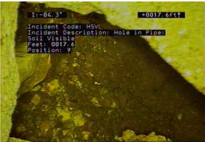
HSV - Hole in Pipe: Soil Visible @ 17.6 ft.
