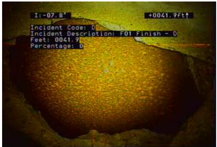
D - Pipe Deformed @ 41.9 ft.
