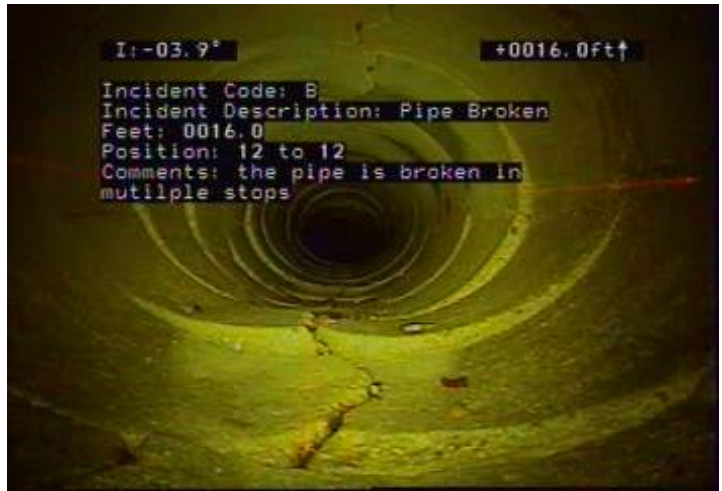
B - Pipe Broken @ 16.0 ft. the pipe is broken in mutilple stops
