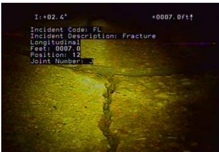
FL - Fracture Longitudinal @ 7.0 ft.
