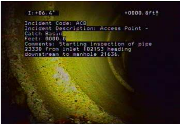
ACB - Access Point - Catch Basin @ 0.0 ft. Starting inspection of pipe 23330 from inlet 102153 heading downstream to manhole 21636.
