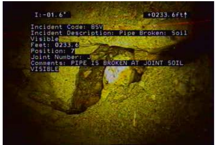
BSV - Pipe Broken: Soil Visible @ 233.6 ft. PIPE IS BROKEN AT JOINT SOIL VISIBLE
