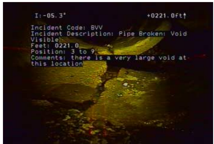
BVV - Pipe Broken: Void Visible @ 221.0 ft. there is a very large void at this location
