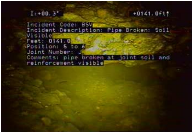
BSV - Pipe Broken: Soil Visible @ 141.0 ft. pipe broken at joint soil and reinforcement visible
