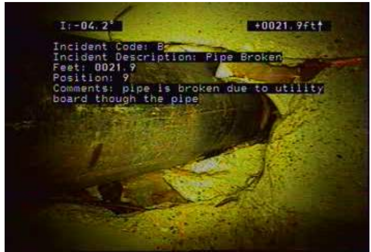
B - Pipe Broken @ 21.9 ft. pipe is broken due to utility board though the pipe
