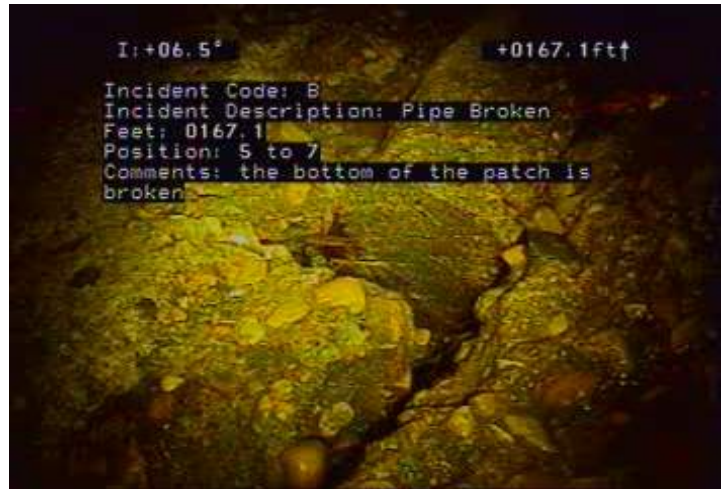
B - Pipe Broken @ 167.1 ft. the bottom of the patch is broken
