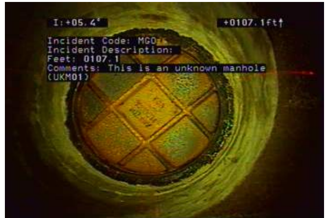
MGO - General Observation @ 107.1 ft. This is an unknown manhole (UKM01) we located this location at 407 W Annie St
