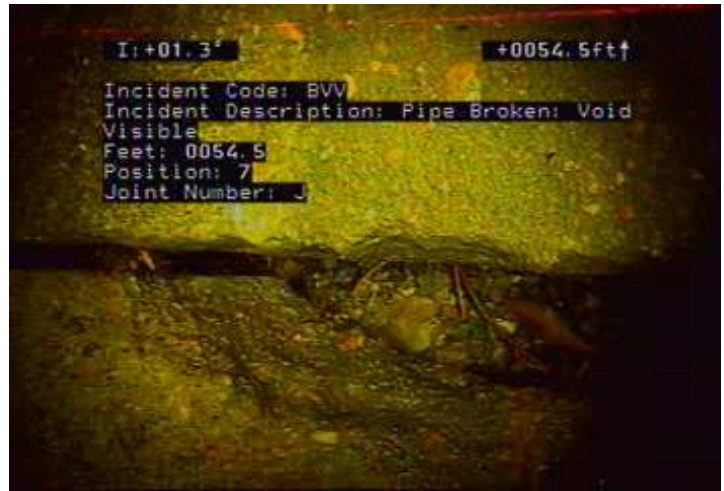
BVV - Pipe Broken: Void Visible @ 54.5 ft.
