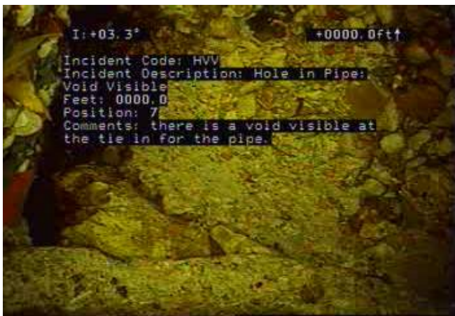
HVV - Hole in Pipe: Void Visible @ 0.0 ft. there is a void visible at the tie in for the pipe.
