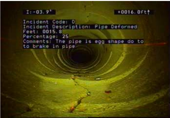
D - Pipe Deformed @ 15.8 ft. The pipe is egg shape do to to brake in pipe
