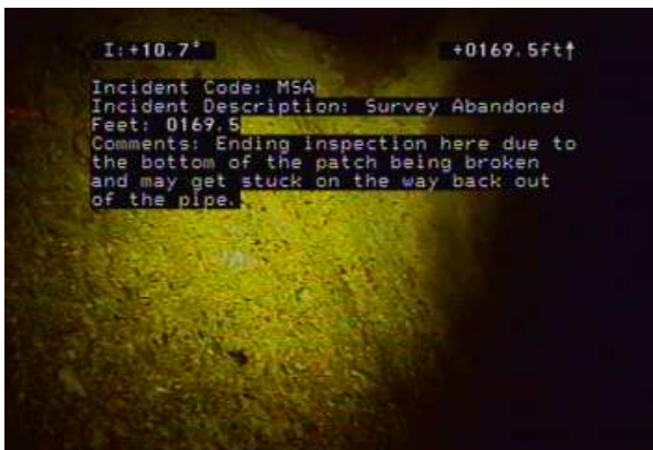
MSA - Survey Abandoned @ 169.5 ft. Ending inspection here due to the bottom of the patch being broken and may get stuck on the way back out of the pipe.
