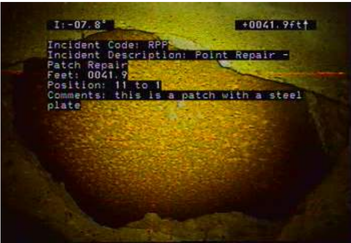
RPP - Point Repair - Patch Repair @ 41.9 ft. this is a patch with a steel plate
