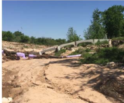
Pedestrian bridge failure due to erosion at Roy G. Guerrero Park
