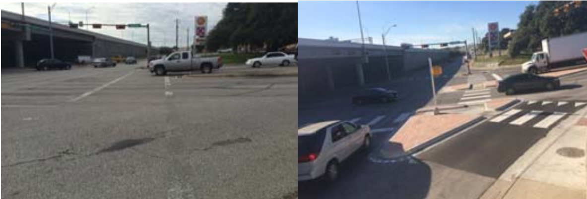
US 183 SR at Cameron Road: Before condition US 183 SR at Cameron Road: After safety improvements
