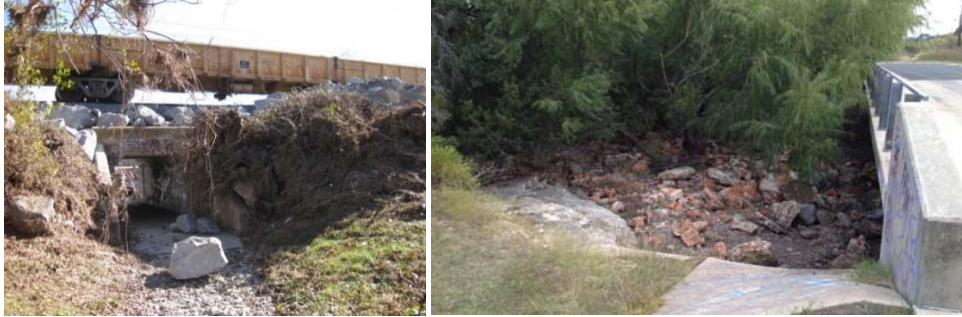
Undersized creek crossing of Walnut Creek near Whispering Valley Drive
