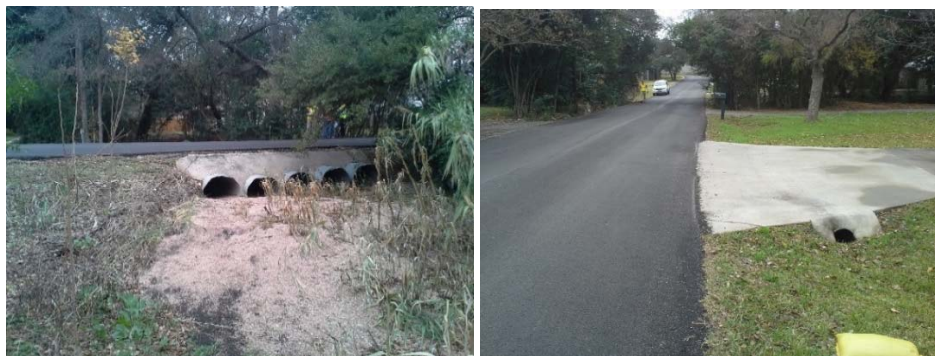
Undersized infrastructure in the Oak Park and Oak Acres subdivisions
