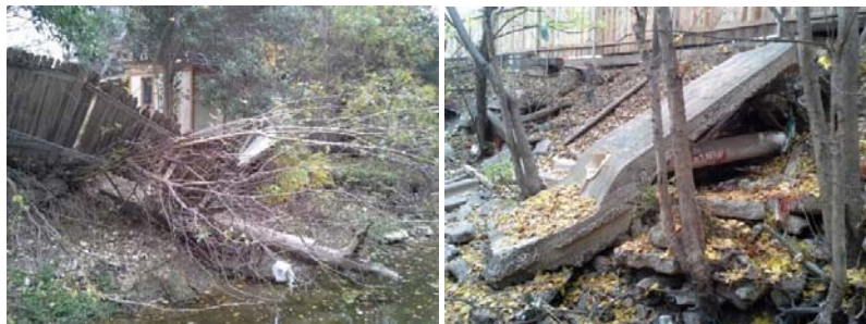
Channel erosion on Little Walnut Creek threatens private fences (left) and storm drain outfalls (right)
