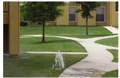
Broken spray head
